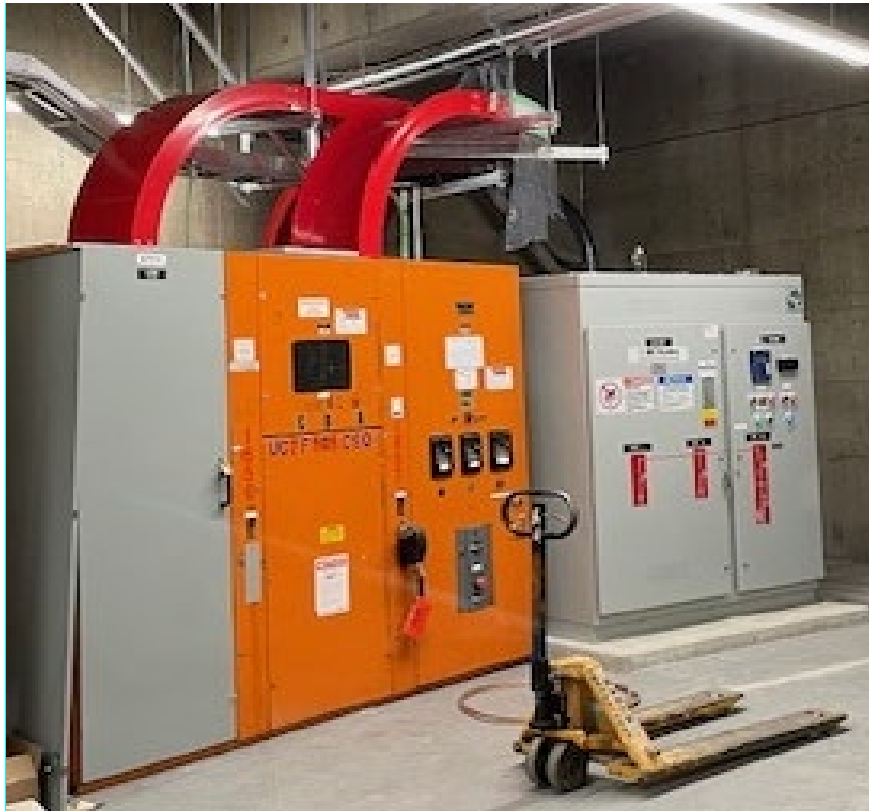
Figure 9-1 – Old 12.5 kV dual radial switchgear next to new 3-way dead-front switchgear
