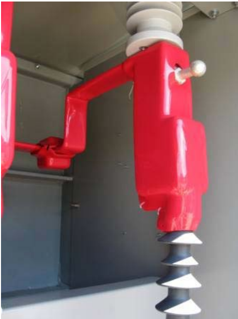
Figure A3-3 – BC Hydro cable termination with ground stud boot removed (live-front)
