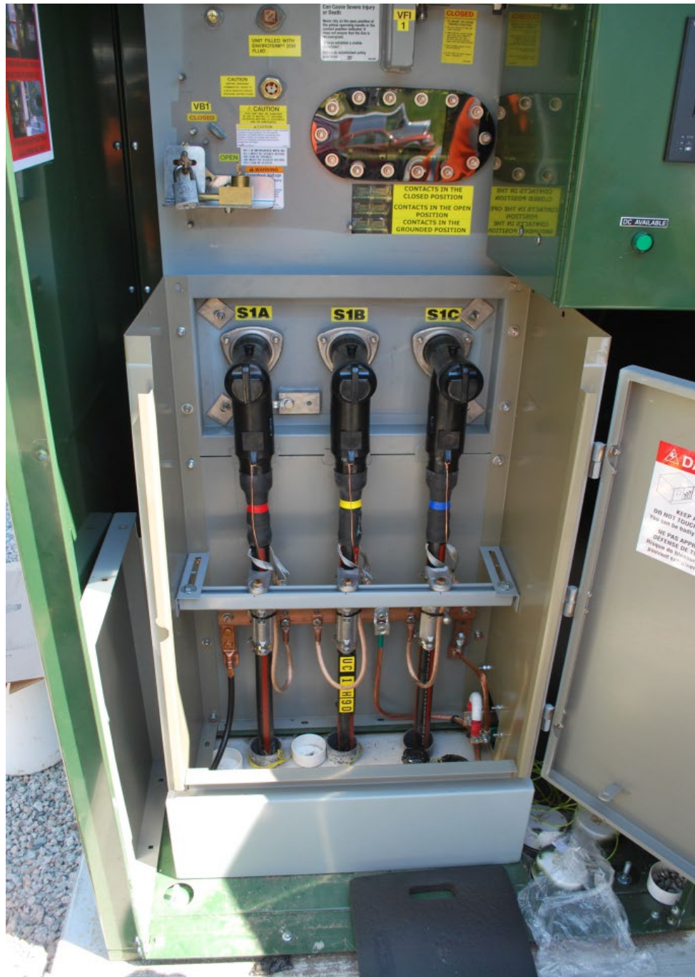
Figure A3-11 – Close-up of dead front BC Hydro utility service cable compartment with terminators, cable supports, and grounding
