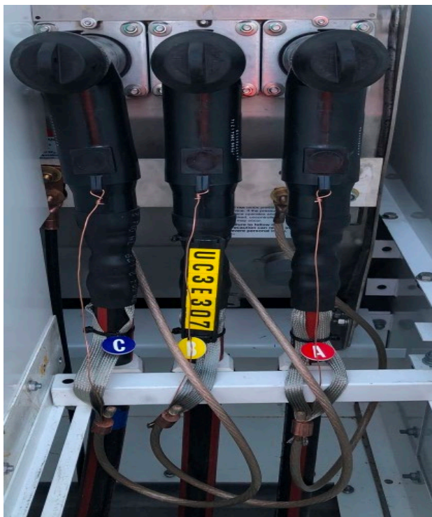
Figure A3-19 – BC Hydro utility cable compartment and cable supports and grounding
