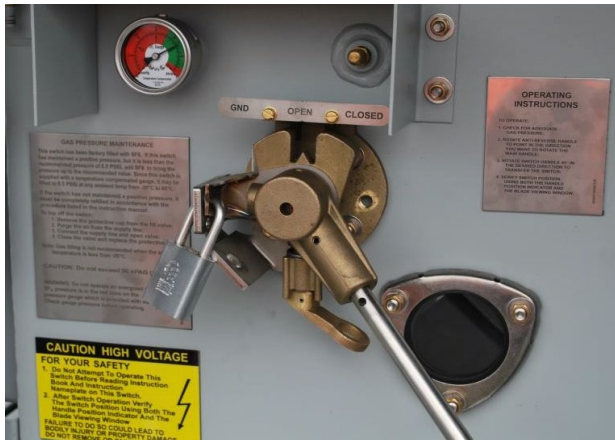
Figure A3-15 – BC Hydro grounding position lock
