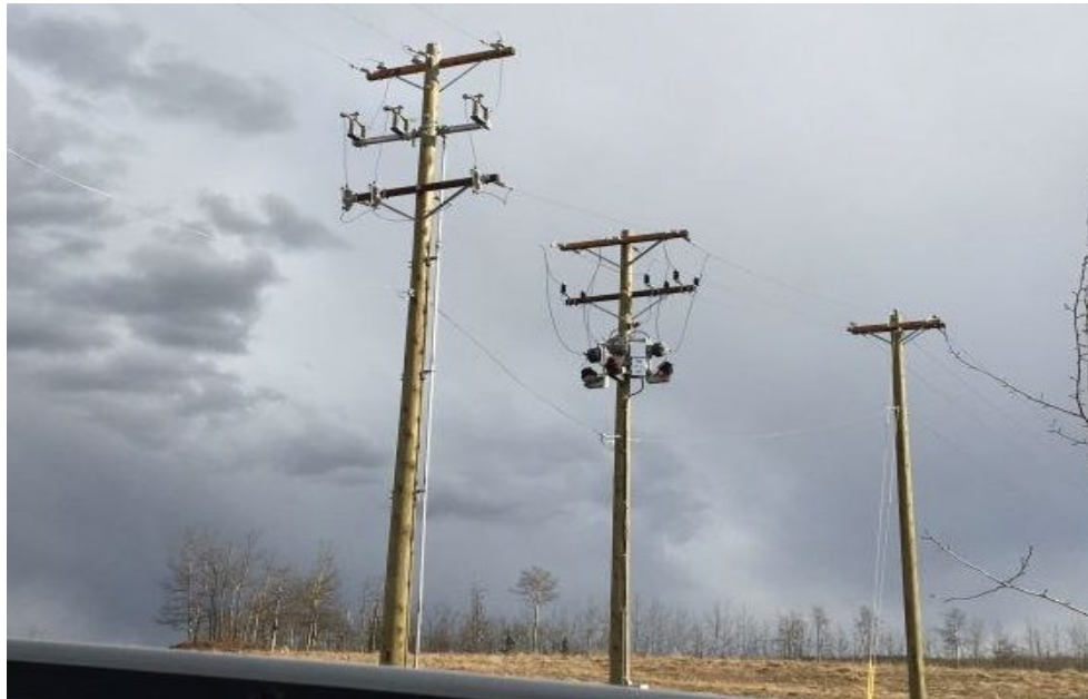
Figure A3-7 – Customer service switch and O/C protection on first pole and BC Hydro primary revenue metering on second pole
