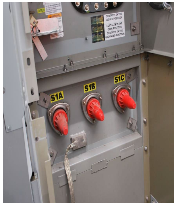
Figure A3-9 – Dead-front kiosk both doors open showing grounding switch above and service cable bushings below
