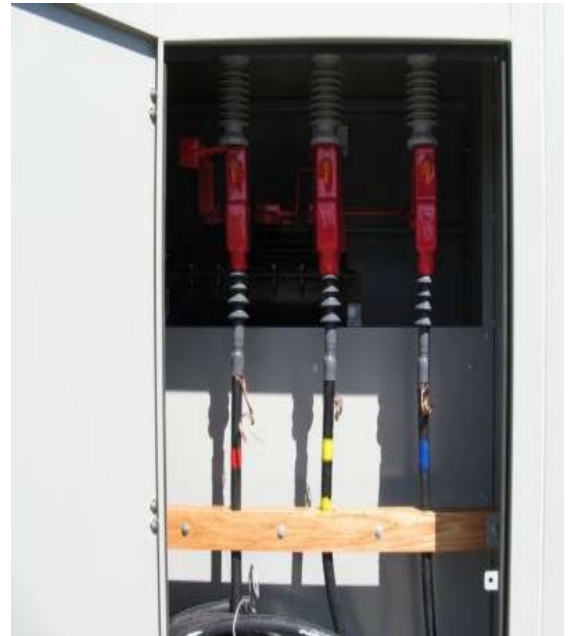
Figure A3-2 – Utility service cable compartment showing disconnect switch and primary bus work (live-front)
