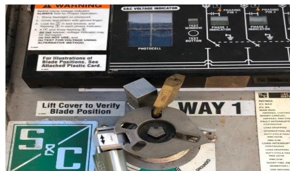
Figure A3-20 – BC Hydro grounding position lock
