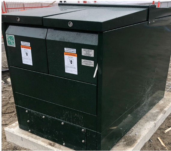
Figure A3-17 – Dead-front primary service kiosk by S&C Electric showing BC Hydro as way 1 and customer service main as way 2
