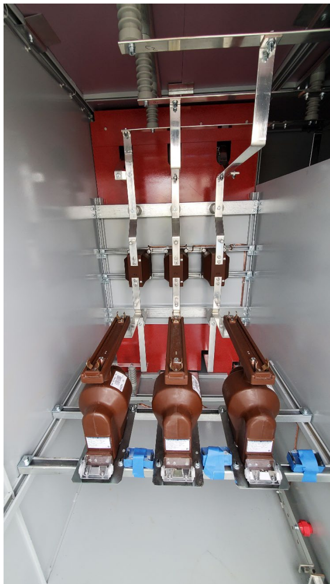
Figure A3-5 – Primary revenue metering compartment
