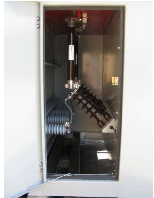
Figure A3-4 – Customer-owned primary service fuse compartment
