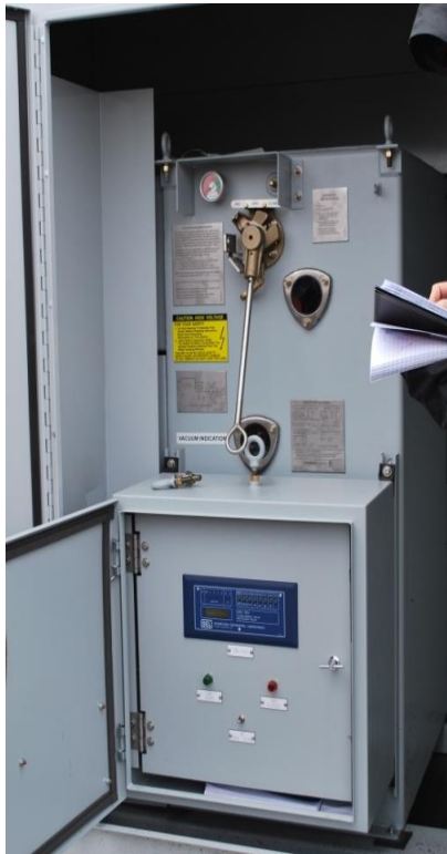
Figure A3-12 – Dead front primary service kiosk by Power Systems Technology showing service main
