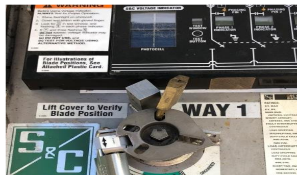
Figure A3-20 – BC Hydro grounding position lock
