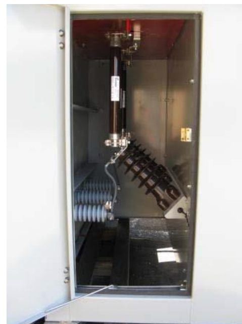
Figure A3-4 – Customer-owned primary service fuse compartment
