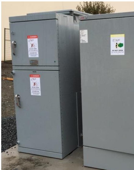
Figure A3-8 – Customer-owned dead-front kiosk with both doors closed
