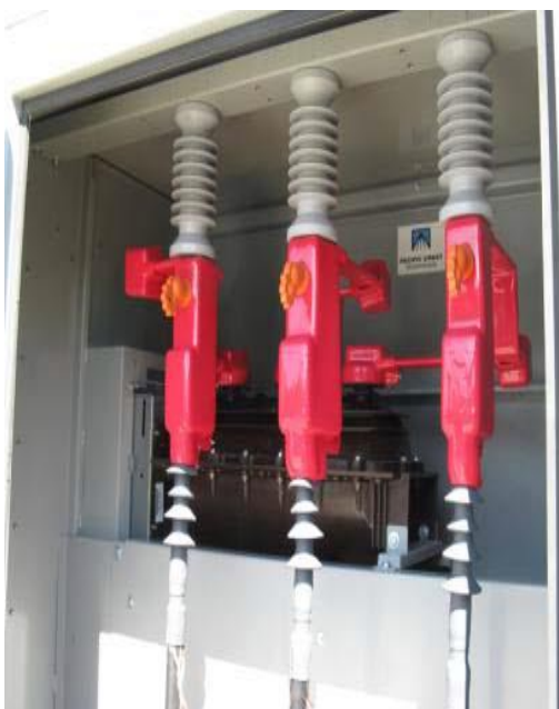
Figure A3-1 – BC Hydro utility service cable compartment (live-front)
