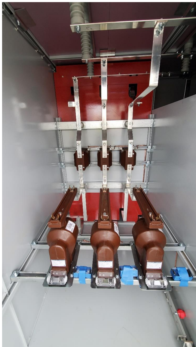
Figure A3-5 – Primary revenue metering compartment
