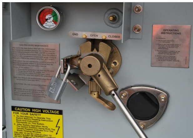
Figure A3-15 – BC Hydro grounding position lock
