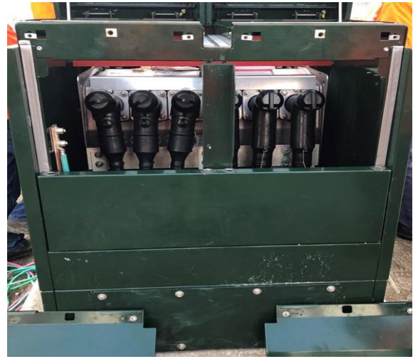
Figure A3-18 – Dead-front primary service kiosk by S&C Electric with BC Hydro as way 1 and customer service main as way 2, covers open
