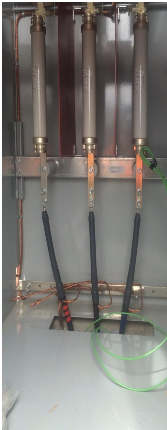
Figure A3-6 – Customer fuse compartment with customer primary service cable terminations
