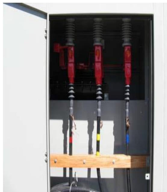
Figure A3-2 – Utility service cable compartment showing disconnect switch and primary bus work (live-front)
