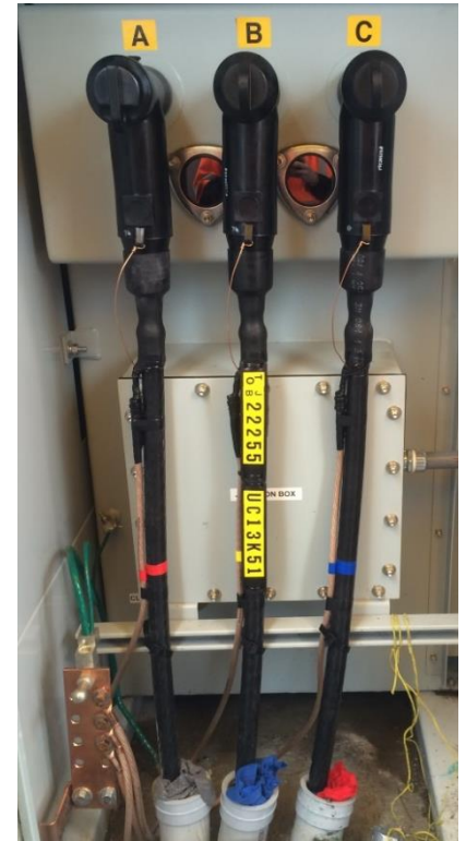
Figure A3-14 – BC Hydro utility cable compartment and cable supports and grounding
