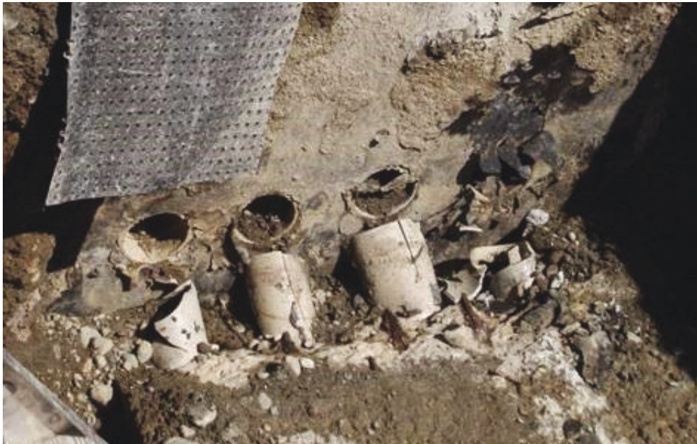
Figure 1 – Service ducts sheared due to settlement and lack of rebar reinforcement
