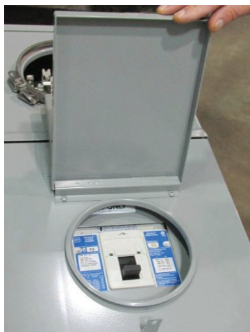
Figure 9 – Customer breaker with lockable cover
