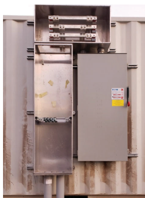
Figure 2 – Unacceptable loadbreak switch
