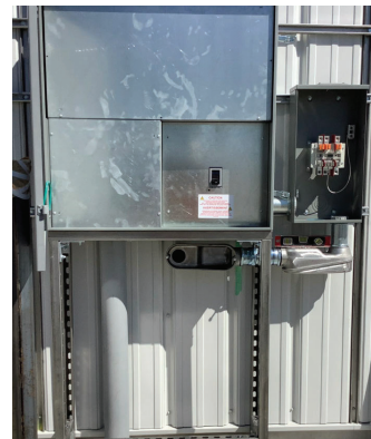
Figure 3 – Acceptable service main breaker
