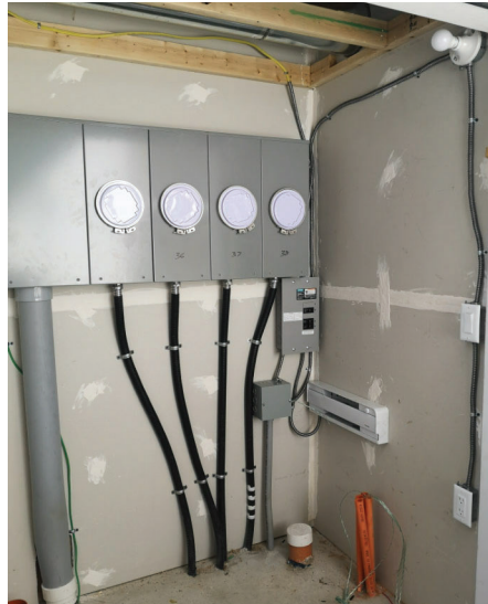
Figure 1 – Acceptable commercial meter closet inside building
