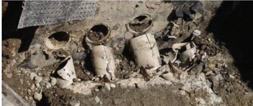
Figure 1 – Service ducts sheared due to settlement and lack of rebar reinforcement
