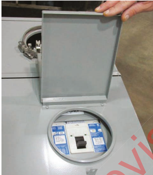
Figure 9 – Customer breaker with lockable cover
