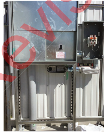
Figure 3 – Acceptable service main breaker
