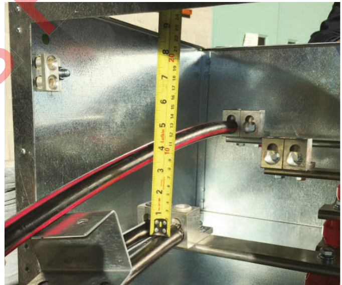
Figure 11 – Phase cables staggered over neutral
