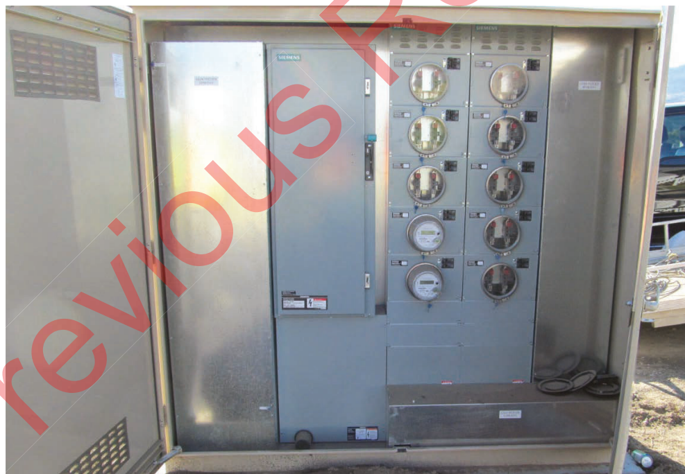
Figure 14 – Unacceptable revenue meter centre kiosk with fused loadbreak switch
