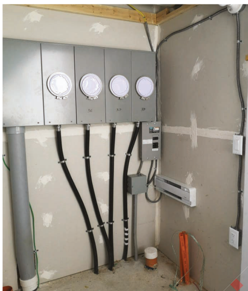
Figure 1 – Acceptable commercial meter closet inside building
