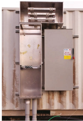
Figure 2 – Unacceptable loadbreak switch
