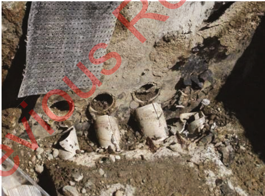
Figure 1 – Service ducts sheared due to settlement and lack of rebar reinforcement
